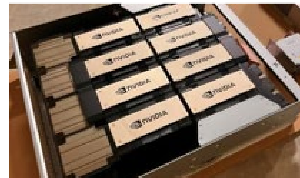
October 2023: Setting up GPU servers at Ishikari Data Center
